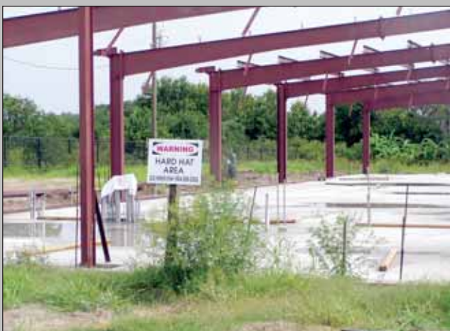
COURTESY UCF ATHLETICS Construction of the $2.5 million UCF Intercollegiate Rowing Center on Lake Pickett Road is underway. The 18,000 sq. ft. facility is set to be completed mid-September.
